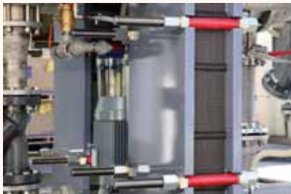
Two heat exchanger units
