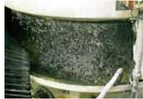
Algae grows on the surface of a cooling tower side.
