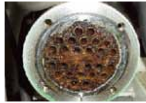
Rust in pipes of a oil-cooler.
