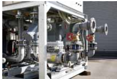
Two lines of piping for machines
